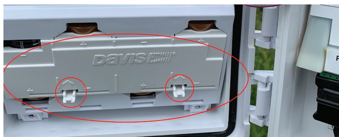
Figure 2: Battery cover inside node door.
